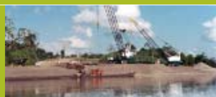
Cranes digging vast quantities of construction materials from the Urubamba river bank along the right of way for the Camisea gas pipeline in Peru, August 2002.
