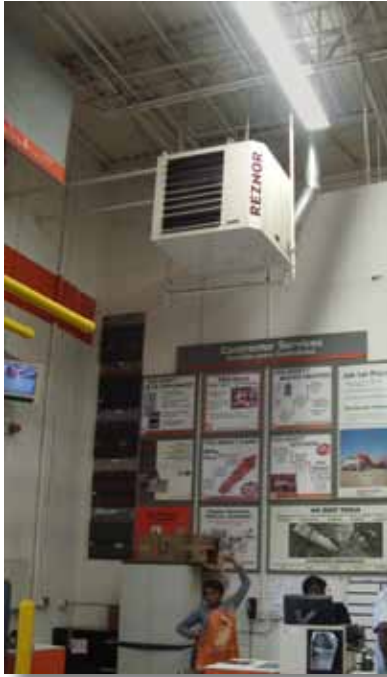
Reznor Model UDAP Gas-Fired Unit Heater in a Retail Store
