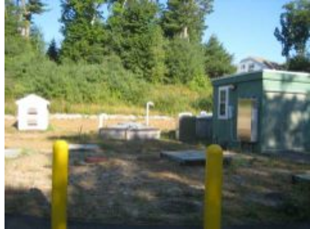
Bioclere units and Control building
