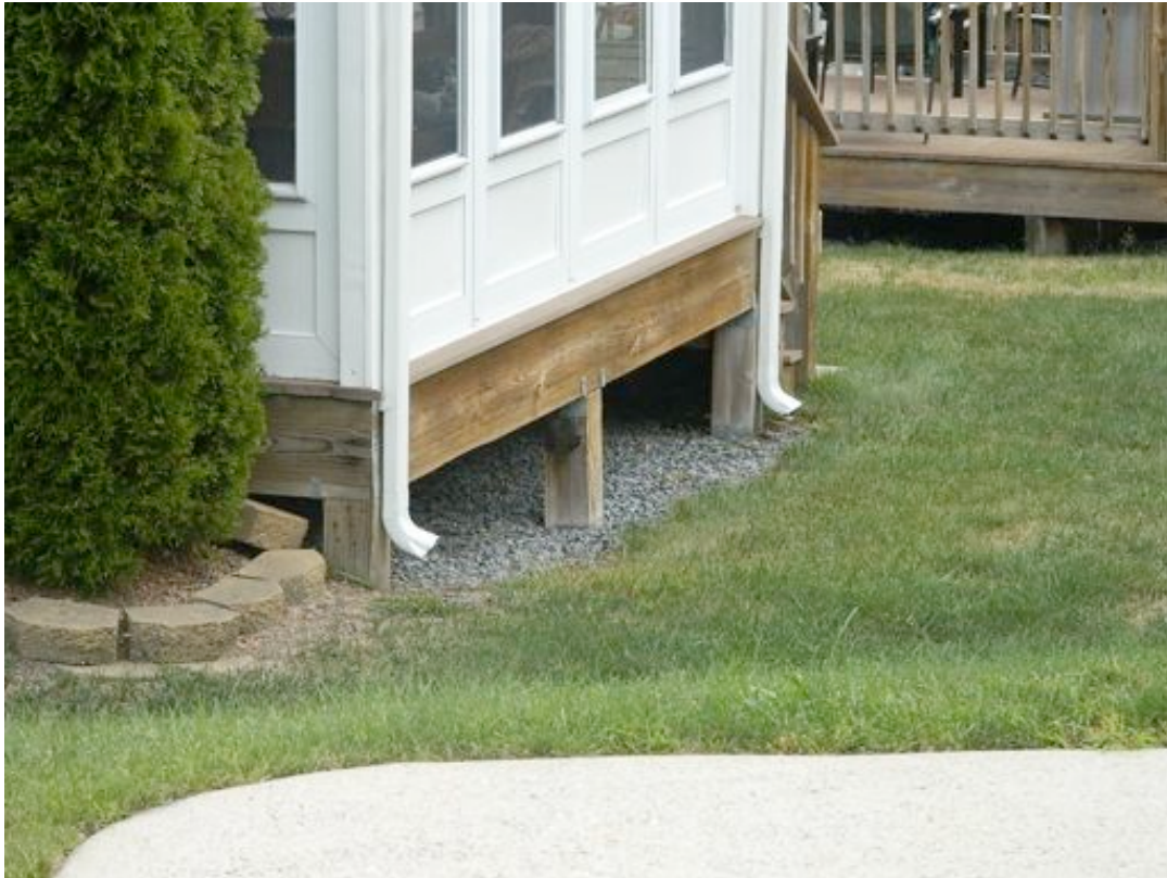
THE REAR GUTTERS SPILL TO GRADE
