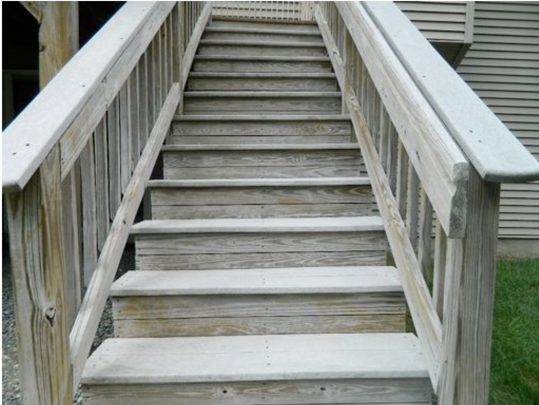
SETTLING DECK STEPS AT THE REAR DECK OF 22 SCHOONER
