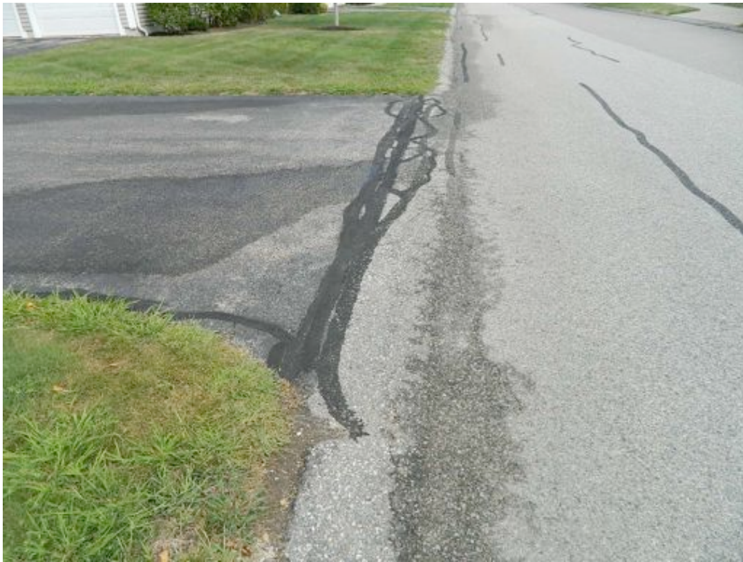
SEALED CRACKS WERE FOUND AT THE END OF MOST DRIVEWAYS
