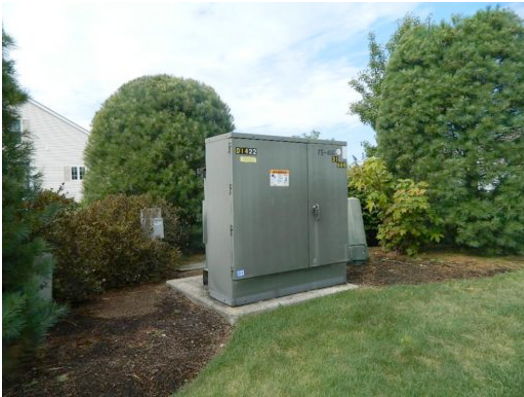
TYPICAL ON-SITE TRANSFORMER
