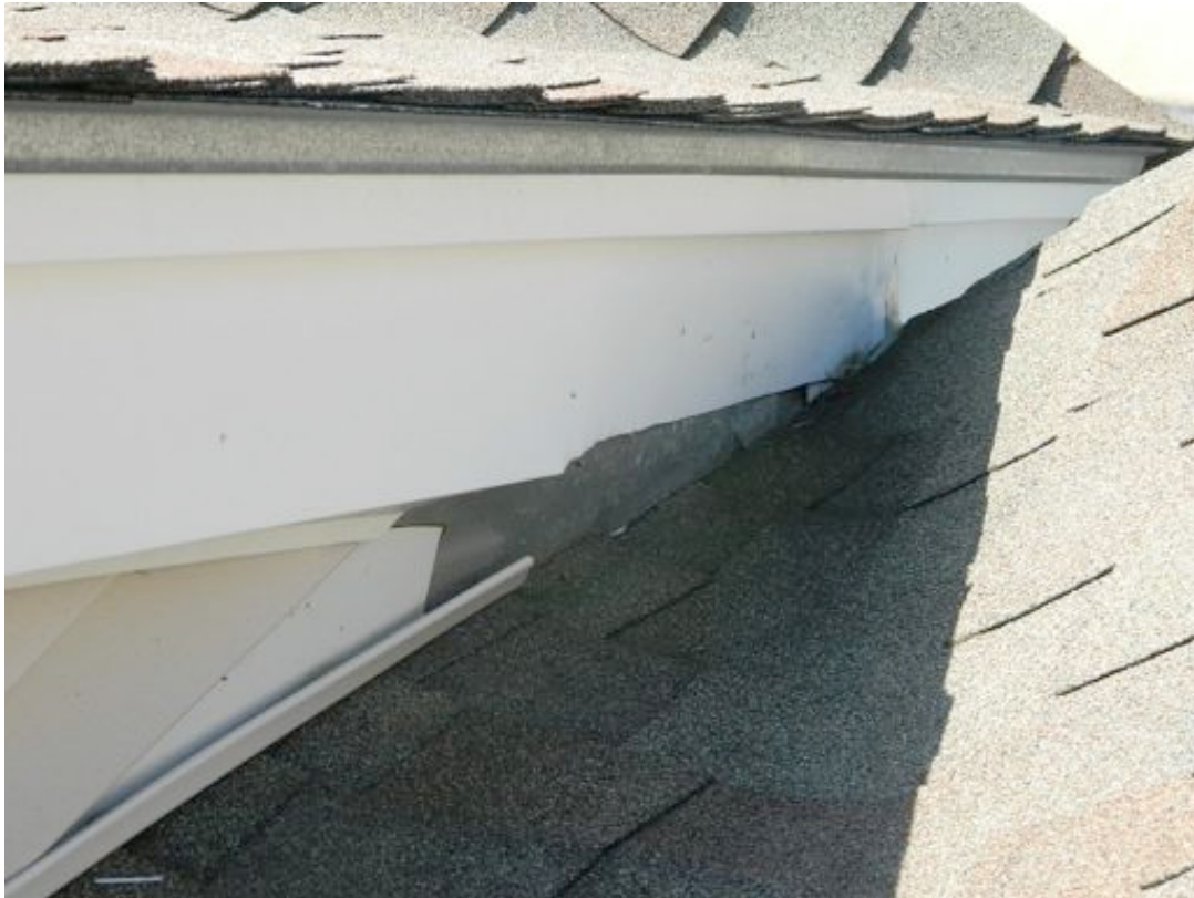
QUESTIONABLE FLASHING DETAILS WERE FOUND WHERE SOME UNITS MERGE
