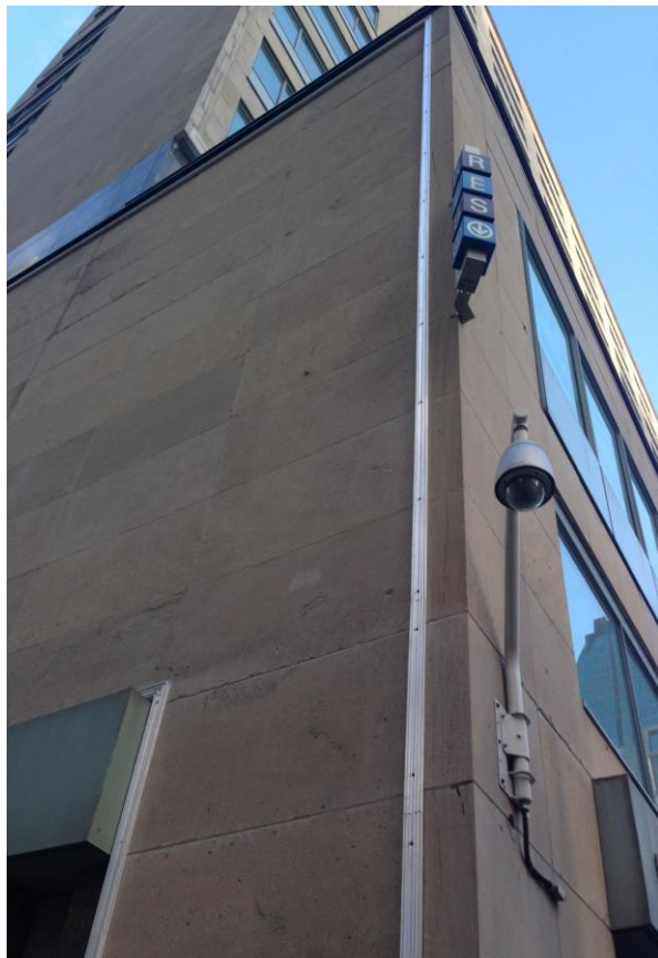
TS44 extrusions installed on a downtown building. Next step will be to stretch the graphic.
