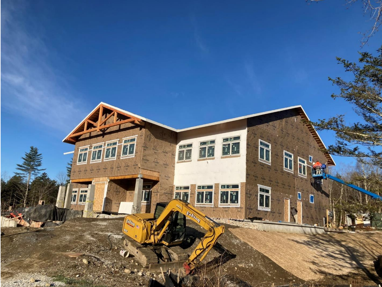
Photo 3 Progress photo of the new Supervisors Office in Mendon. USDA Forest Service photo.
