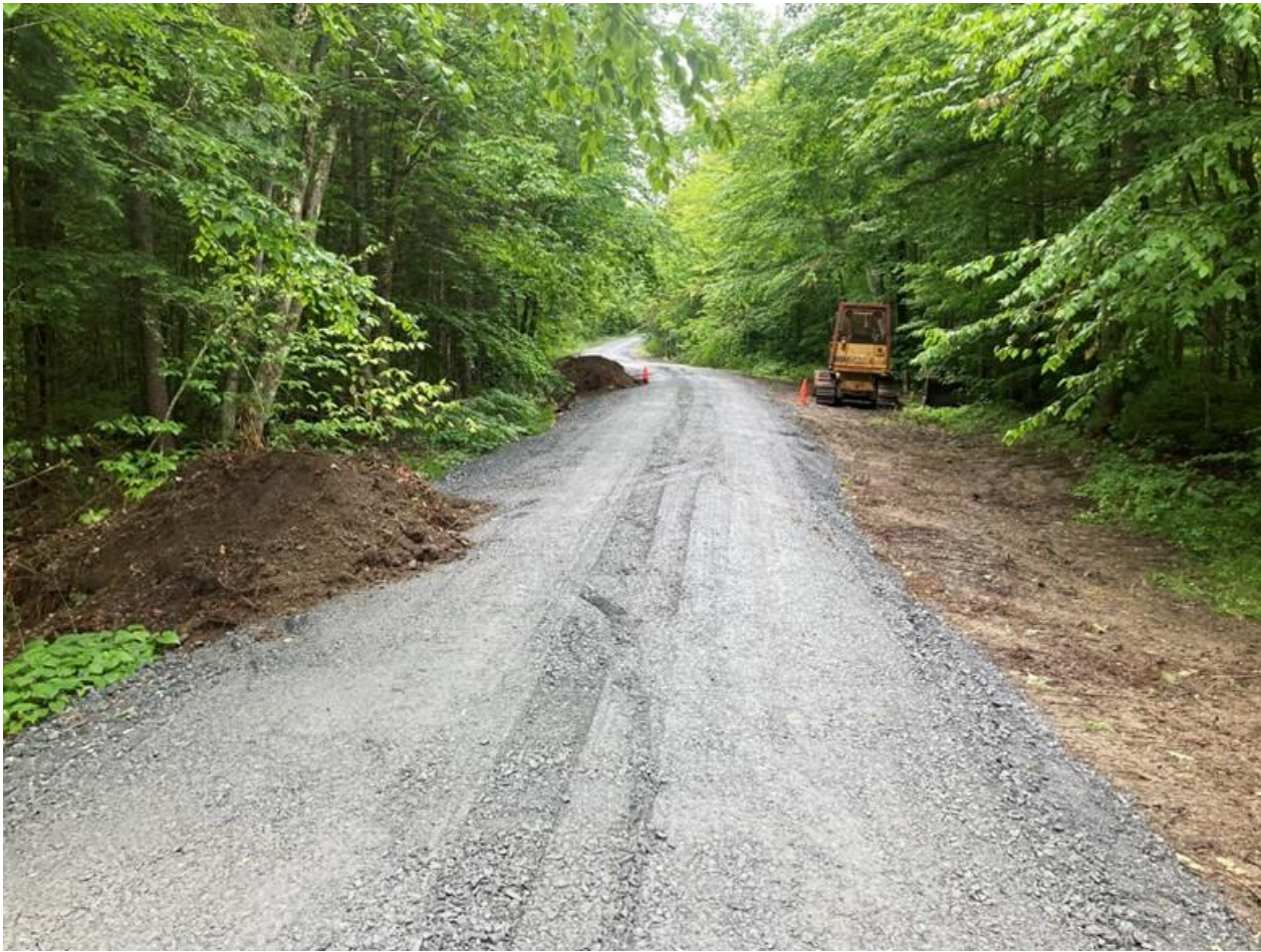
Photo 4 Construction work being done on the Forest Road 39 in Hancock. USDA Forest Service photo.
