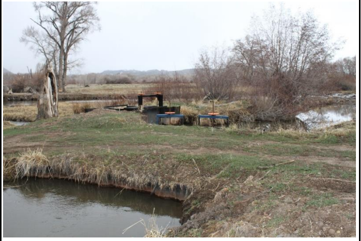
Headgate outlet and adjustment gates
