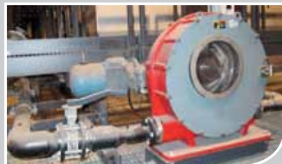
Washing liquid circulation pumps in Talvivaara mine.
