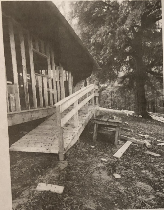
A new designed and built wheel-chair accessible ramp that will help provide access to one of the buildings on the campus that serves as a storage facility and concession area.
