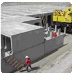
Subsurface infiltration basin in Rancho Mirage, CA. Photo courtesy of RGA Landscape Architects.
