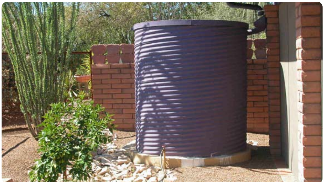
This rainwater cistern installed at a residence in Tucson, Arizona supplies water for citrus trees and a small vegetable garden, as well as native plants. Photo courtesy of Technicians for Sustainability.
