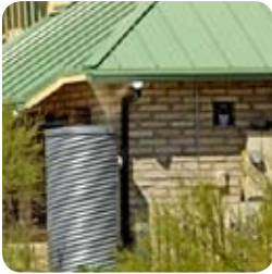
Active rainwater harvesting in Tucson, AZ.
