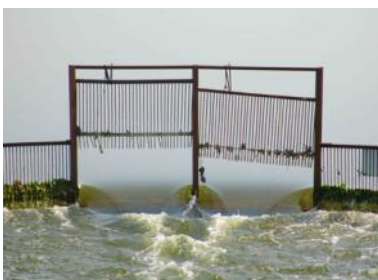
← Juice's modification in action. With the panels raised, water flows freely out of the upper lakes. Note how the adjacent panels are clogged with weeds and debris.
