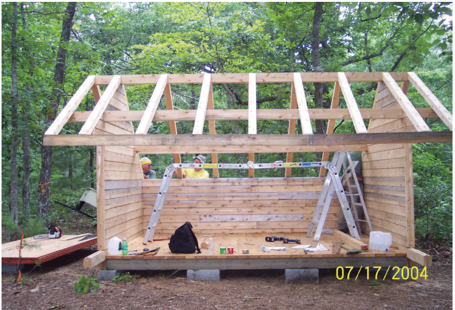
Construction of the Davis Mountain Shelter along the Pinhoti Trail in Alabama.
