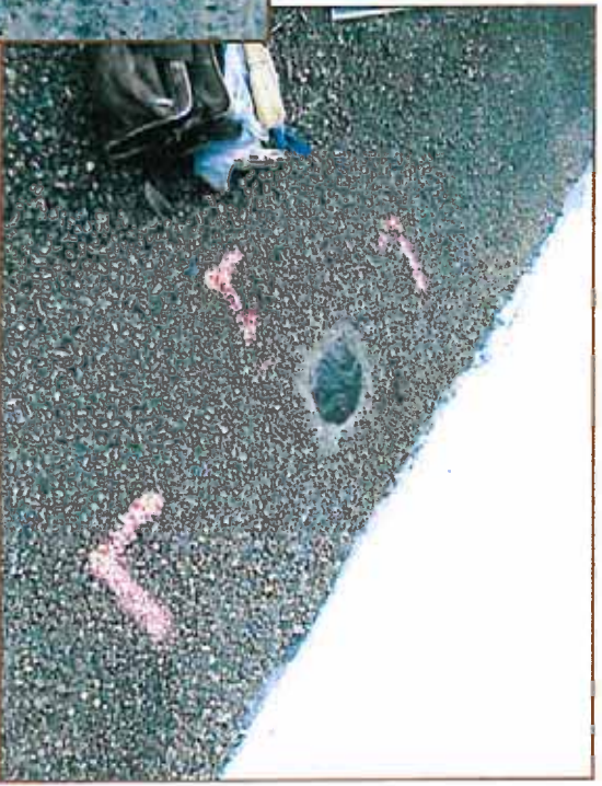
Photo 21 – View of anomaly of wet perlite under BUR.
