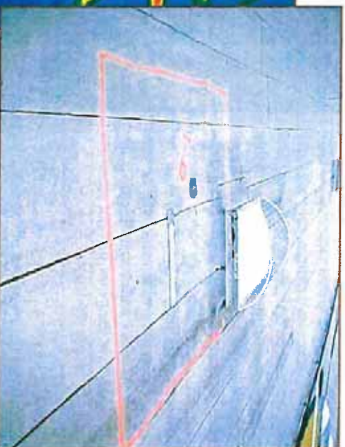
Photograph 6: View of anomaly of wet ISO under modified-bitumen membrane.
