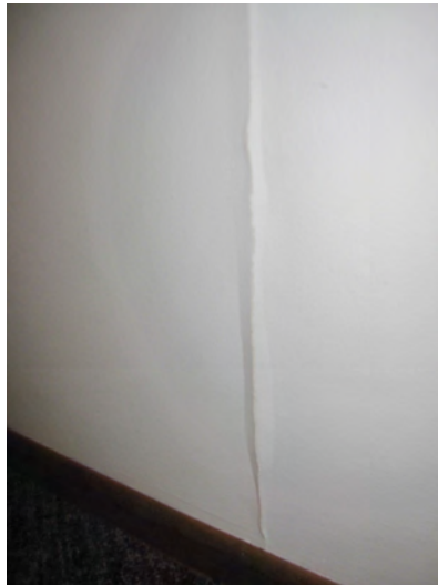
Vertical ridging at east corridor of the 2 nd Floor.
