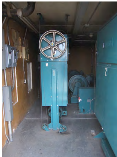
Elevator equipment in the penthouse.
