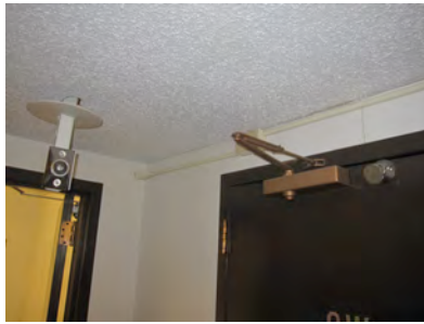
Magnetic hold open attached to a ceiling mounted bracket which needs to be resecured and stabilized.
