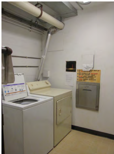
Access panel needed at 9 th Floor Laundry Room.
