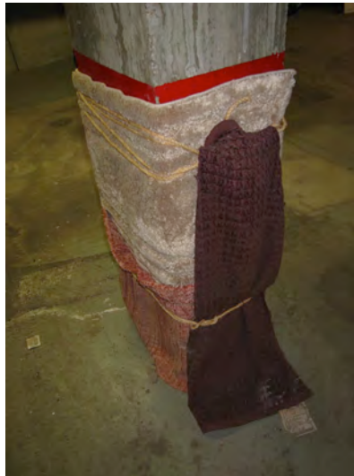
Car door protection at concrete column.
