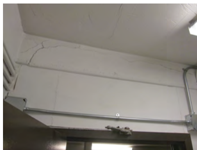
Cracks at 9 th floor laundry room.
