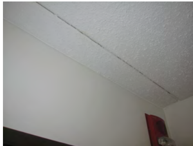
Crack in the sealant joint at the 5 th floor west corridor.
