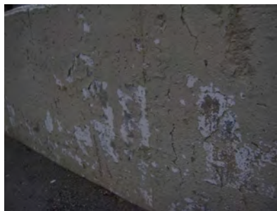
Peeling paint at southwest planter.
