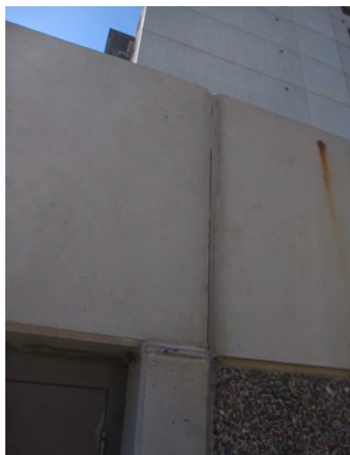
Failed garage level sealant joint, east elevation.
