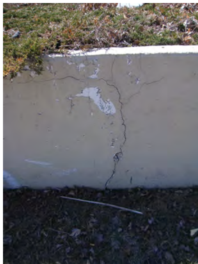
Vertical crack at raised planter wall.
