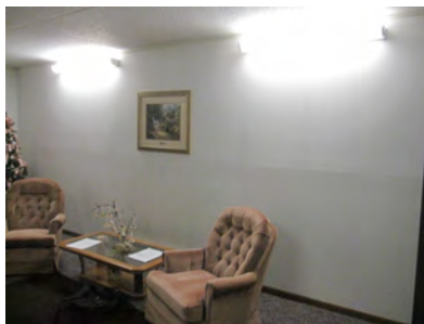
Horizontal ridging at 2 nd floor elevator lobby.
