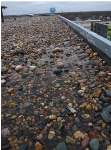
Ponding water in southeast corner of the east tower roof hours after a rain event.
