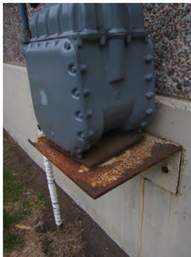
Rusting gas meter bracket.
