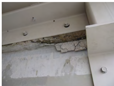
Deteriorated portion of original precast balcony.
