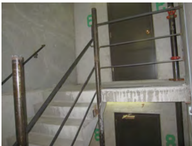
Noncompliant railing/guardrail at east and west tower stairs.
