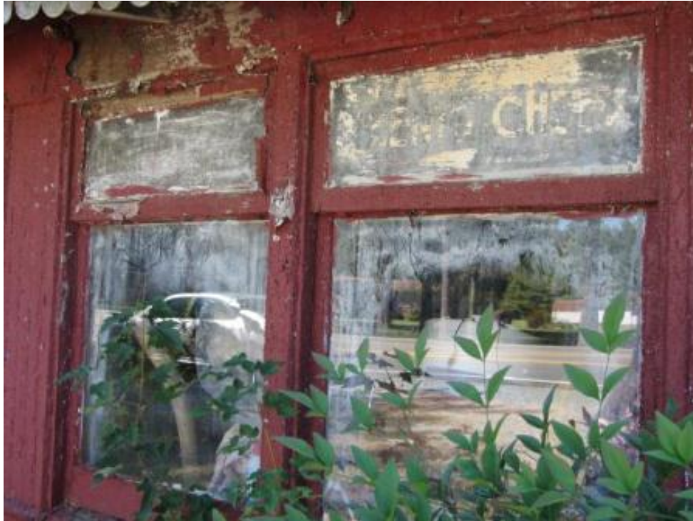
Figure 36. NCDOT Survey #33, Midway Diner (GF-1545), 6270 Burlington Road, Guilford County, windows on north elevation of diner with painted words “pimiento cheese” visible on the right transom.
