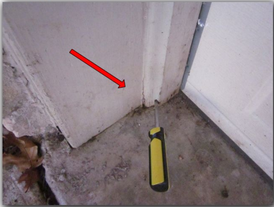
Wood rot at garage trimmer.
