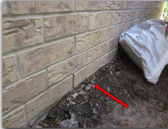
High soil line at right side.
