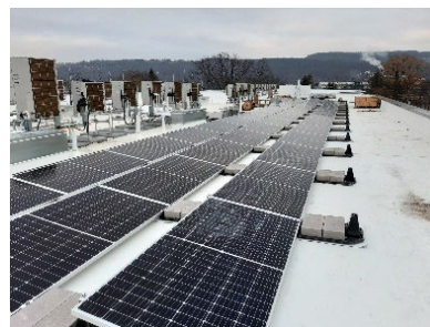
To date, INHS solar arrays have produced about 430 MWh.
