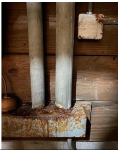
Leak in Boiler room
