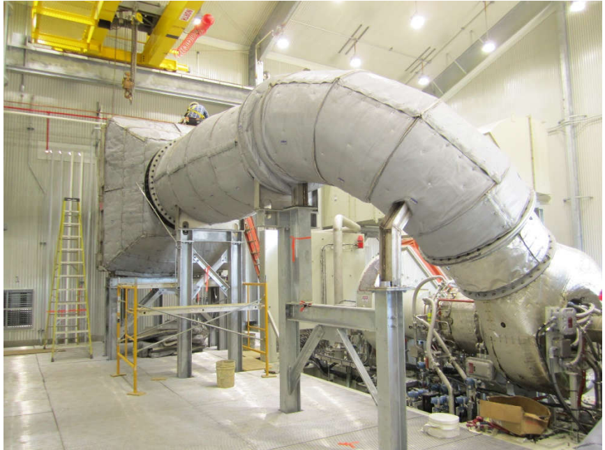
Solar Taurus 60 with oxidation catalyst
