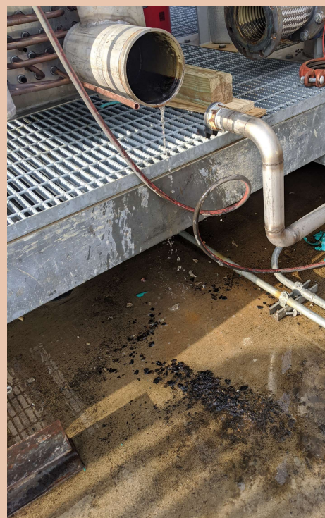
Descaling and Winterization
