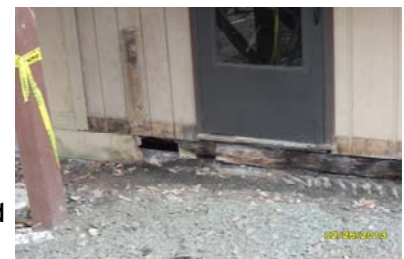
Rotted Box Plate Under A101
