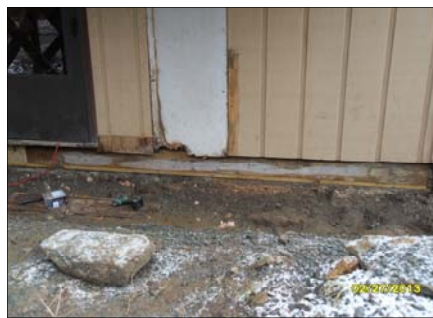
Rotted Box Plate Under A101
