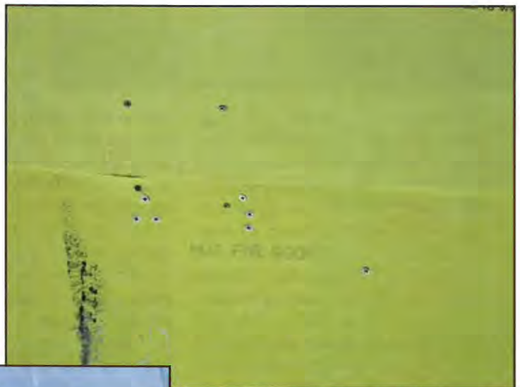
Figure 10 – Improperly positioned fasteners in sheathing.
