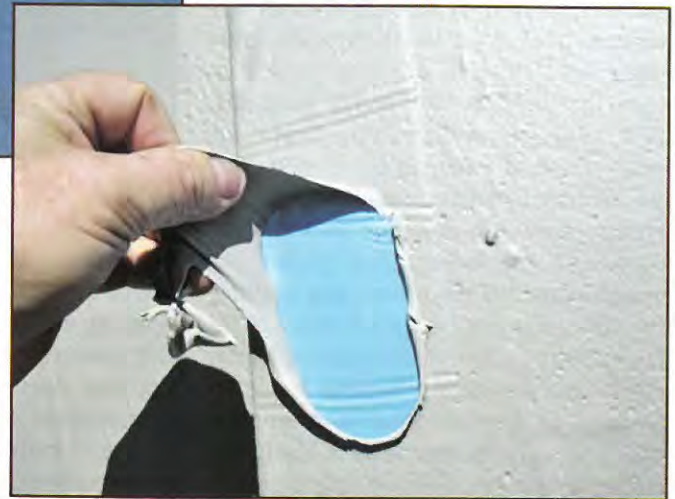
Figure 7 – Delamination of fluid-applied air barrier from transition membrane sheet.
