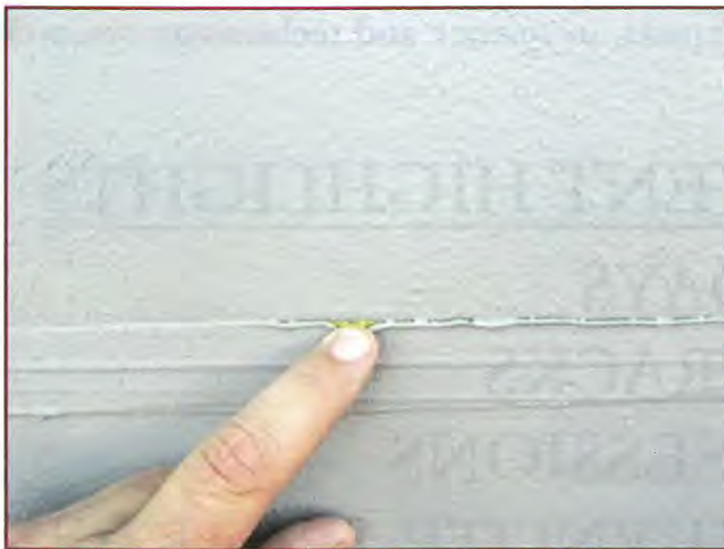
Figure 1 – Exposed face of sheathing along heavy build of sealant at joint.
