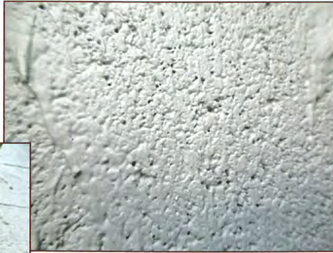
Figure 12 – Voids in fluid-applied air barrier on porous CMU.
