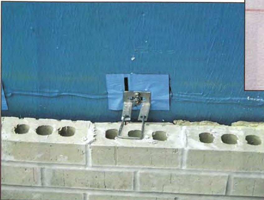
Figure 16 – Cut strip of self-adhered membrane applied on top of fluid-applied air barrier at masonry anchor.
