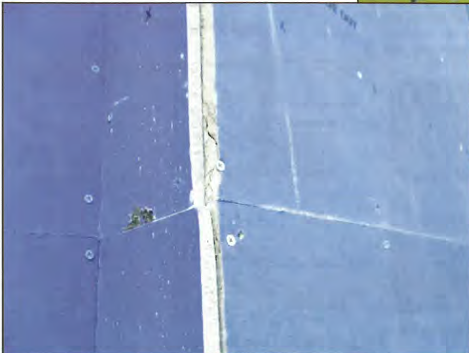
Figure 9 – Exposed gypsum core at outside corner of wall.
