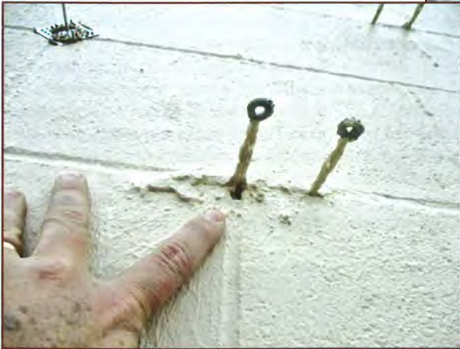
Figure 11 – Void in fluid-applied air barrier at eye hooks of pintle masonry anchor.
