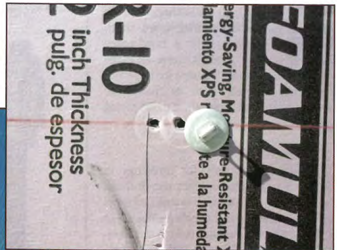
Figure 17 – Multiple screw holes in insulation and underlying WRB.
