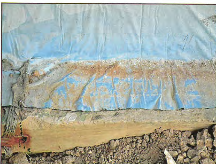
Figure 8 – Soil-contaminated base of wall.
