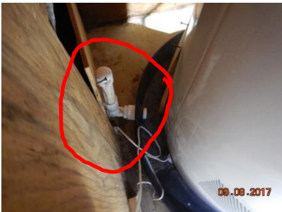
The water heater drain pan drain line has been blocked off.
