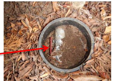
This may a shut off valve for the sprinkler system.
