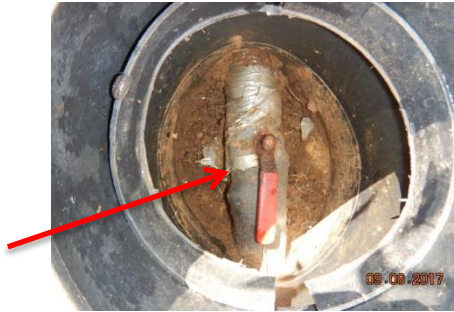
This is the customer shut off valve by the water meter in the front yard.
