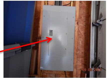
General Electric 200-amp main panel is in the garage.
