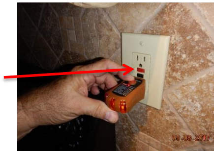
The GFCI outlet next to the range did not trip.
