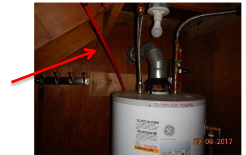
There is no upper and no lower combustion ventilation in the water heater closet.
