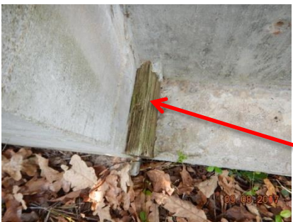
There are form boards in the foundation on the East side of the foundation.
