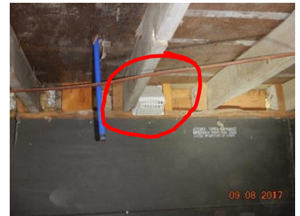
The downstairs washroom exhaust fan vented to the crawl space.
