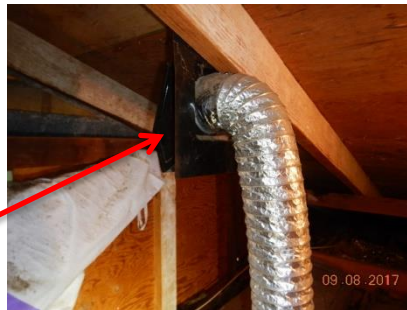
The upstairs washroom exhaust fan vents to the attic.
