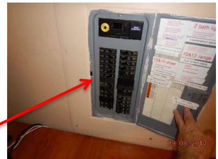
Square D 200-amp sub-panel center with 150-amp main breaker in the Southwest bedroom.
