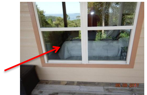
There are windows on the back porch missing screens.
