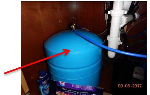
There is an "RO" filter system below the kitchen sink.
