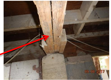
There is old evidence of old WDI in the crawl space.
