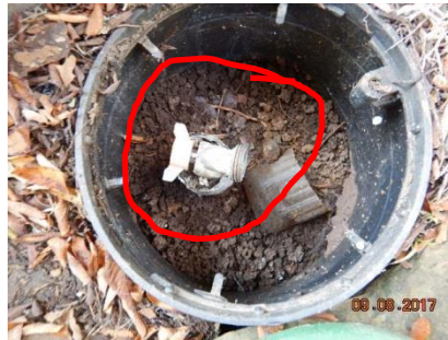
There are two exterior faucets that are missing air gaps.
