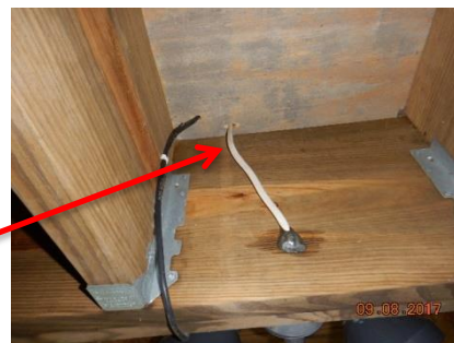
There is exposed romex below the laundry room area floor.
