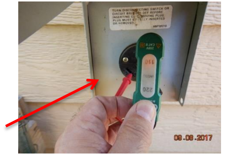
There is an active 30-amp 110v plug at the Southwest exterior corner.
