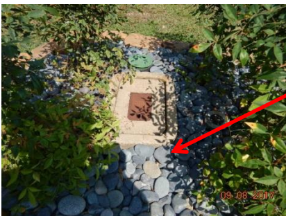
The water meter is by the drive in the flower bed.
