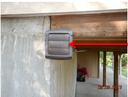
The dryer vented to the East wall.
