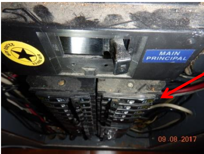
This sub-panel is wired with all copper wiring.
