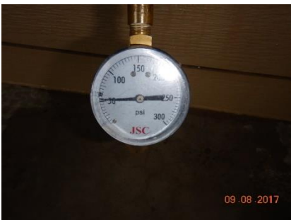
The static water pressure was 55-PSI at the time of this inspection.
