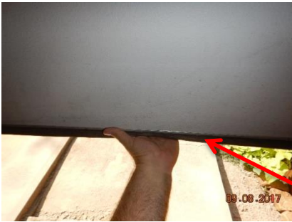
The close tension on the garage door operator is set too high.
