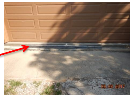
The garage floor to the driveway is missing the apron.
