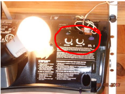
The close tension on the garage door operator is set too high.
