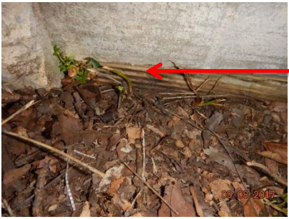
There are form boards in the foundation on the East side of the foundation.
