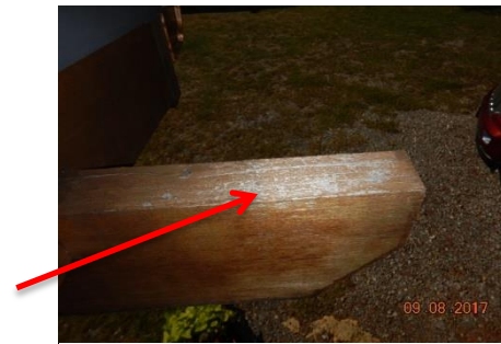
Rafter extension outside the roof edge is missing waterproofing stain.
