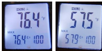
The A/C temperature differential was 18.9°.
