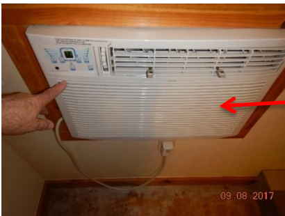
The basement window unit functioned as expected.
