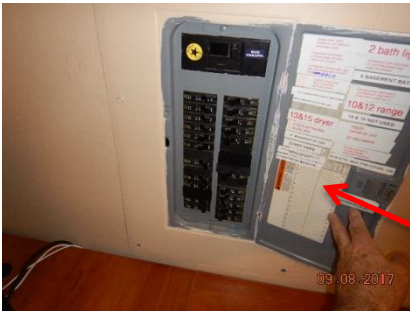
This sub panel appears to be marked on all breakers.
