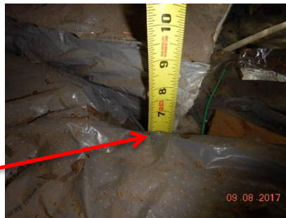
The attic has 6" of rolled insulation throughout the attic area over the main house.
