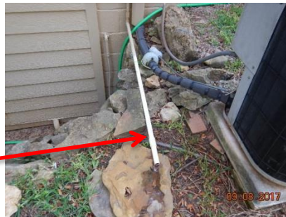
The A/C condensate drain is draining to the West side of the foundation.
