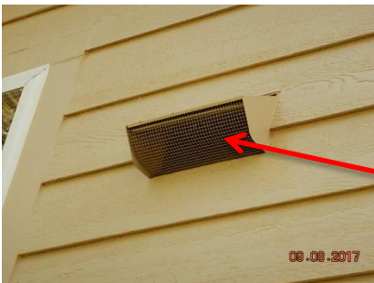
The range hood vents to the West exterior wall.
