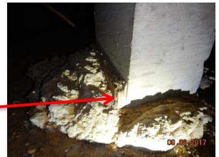
There are form boards imbedded into some piers in the crawl space.
