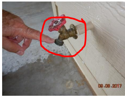
There are two exterior faucets that are missing air gaps.
