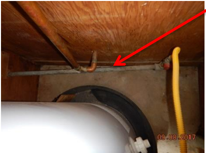
The gas line to the water heater is galvanized iron pipe and should be black pipe.
