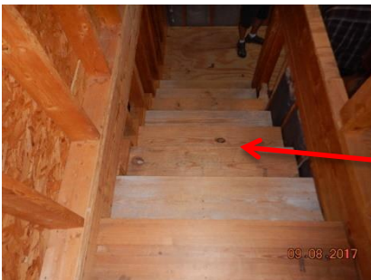
The unfinished stair way will require handrailing when completed.
