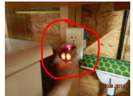
There are some outlets in the garage that are not on a GFCI circuit.
