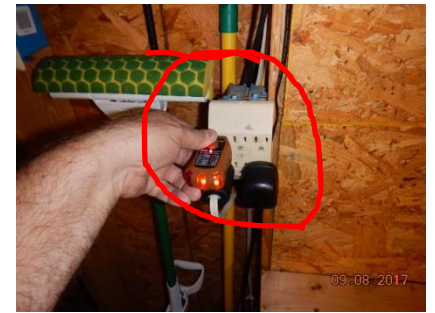
There are some outlets in the garage that are not on a GFCI circuit.
