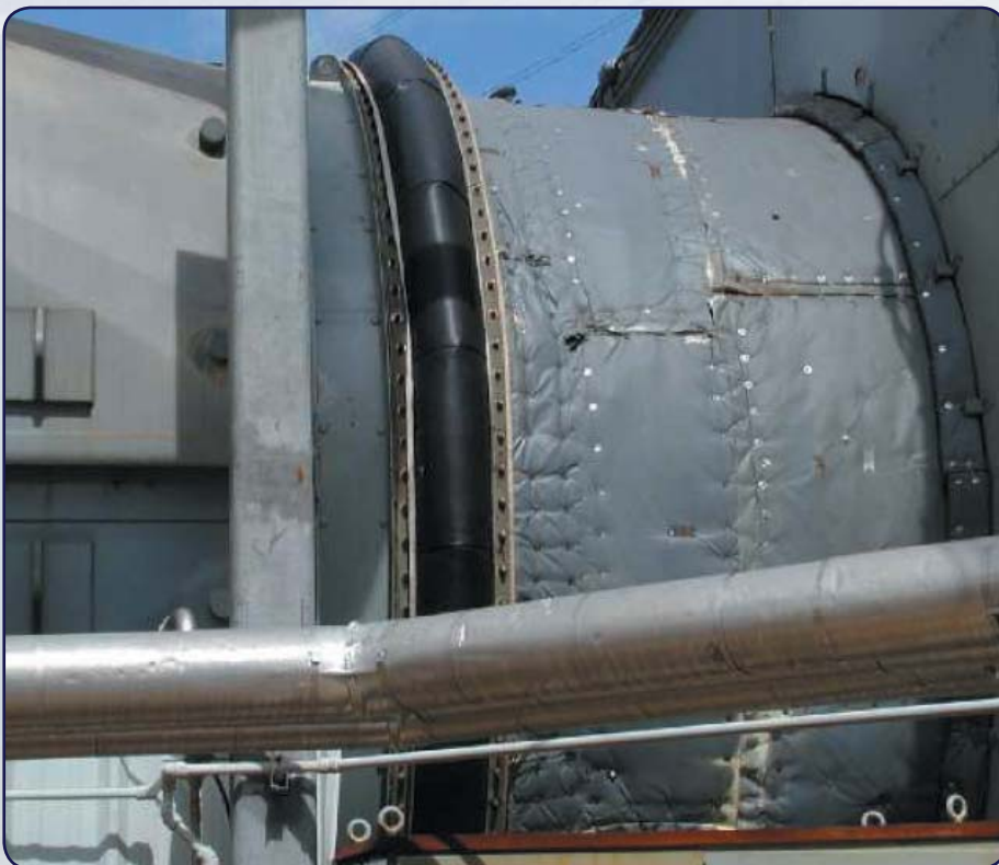
GTEJ installation showing convex belt geometry
