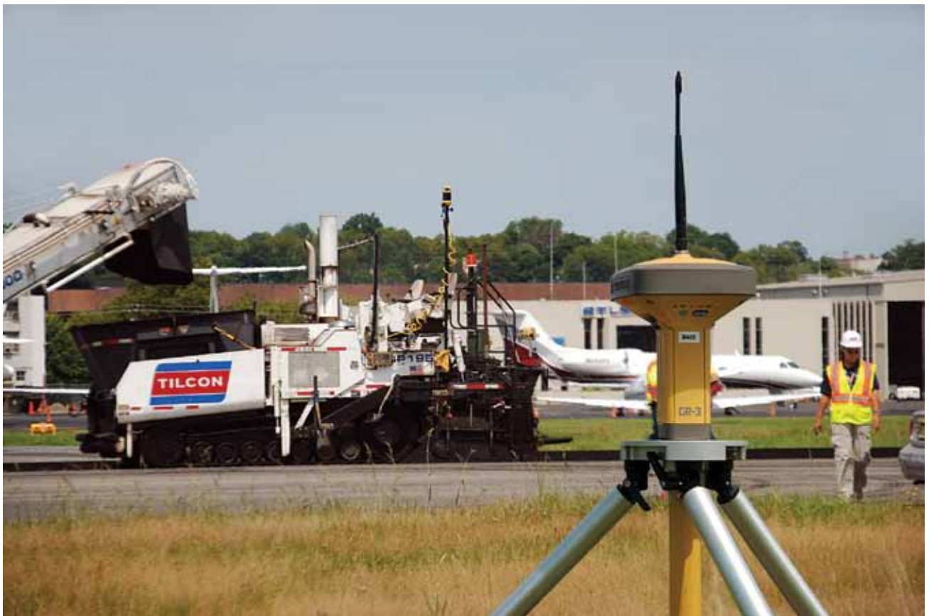
The Topcon GR3 Base Station is positioned close to the paving train.
