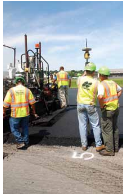
Topcon dealer Jim Cleary checks the grade with the GR3 Survey Rover.
