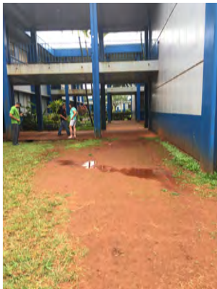
Before: Red clay dirt/mud at entrance
