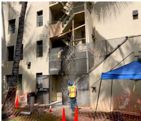
In Progress: work at exterior of building with CPI team and public safety barriers in place
