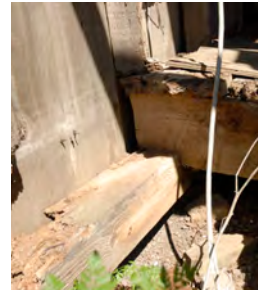
Pre-project: Historic wood foundation rot
