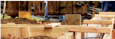
Top: Barn in lifted condition, placement of new concrete foundation; Bottom: foundation formwork
