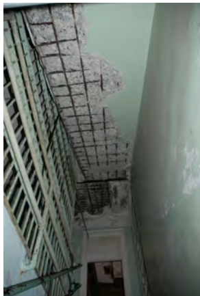
Before: extensive concrete deterioration & steel corrosion, unsafe conditions
