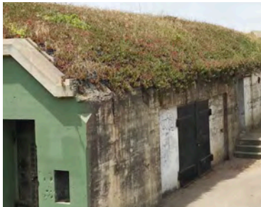
Before: Deteriorated condition, visitor safety compromised
