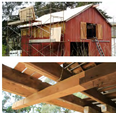
In Progress Top: New roof installation; Bottom: Splicing new wood members to historic
