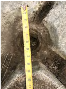
Condition assessment revealed non-functioning drainage pipe
