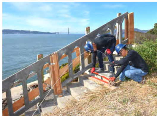
In Progress: Precast concrete panels built off-site, moved & temporarily held in place while team built concrete posts & hand rail in place (Golden Gate Bridge in background)
