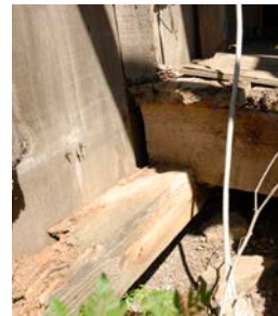
Pre-project: Historic wood foundation rot
