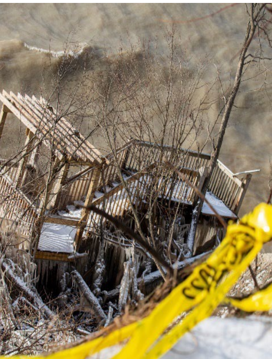
Reparation of damage to Casco Township Nature Preserve Shoreline. January 21, 2020. (Photo Credit: Joel Bissell)
