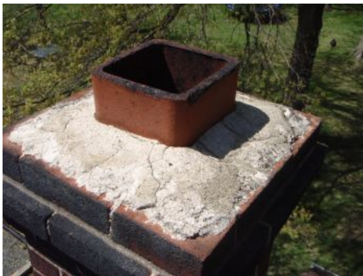
Soot Staining on the Chimney and Flue
