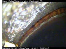
Exposed Joint @ Tee
