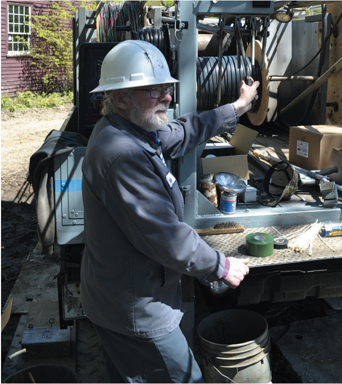
Skip Hodgdon in one of his familiar spots - the back of a drilling rig "putting down hole."
