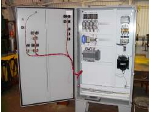
New control panel replaces obsolete controls.
