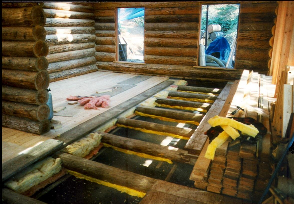
Working On North Side Of East Section (Facing East) This Also Shows The Tucking Of Insulation Into The Space Created By the Curvature Of The Joists As It Meets The Galvanized Mesh
