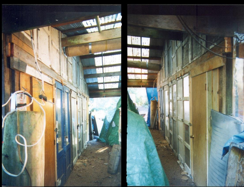
Shop Enclosed North Side With 12 Foot Breezeway For Access Through Shop East And West On Roadway For Vehicles And Tractor
