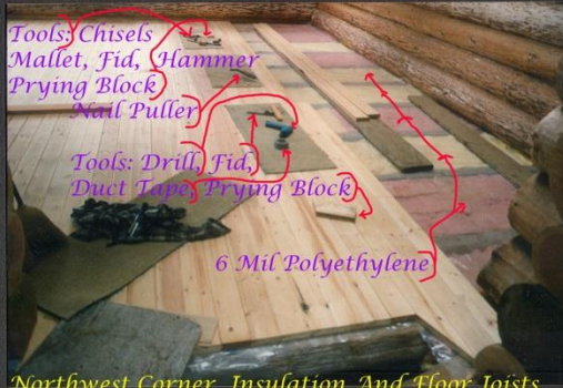
Northwest Corner Insulation And floor Joists Were Covered With 6 Mil Polyethylene.
