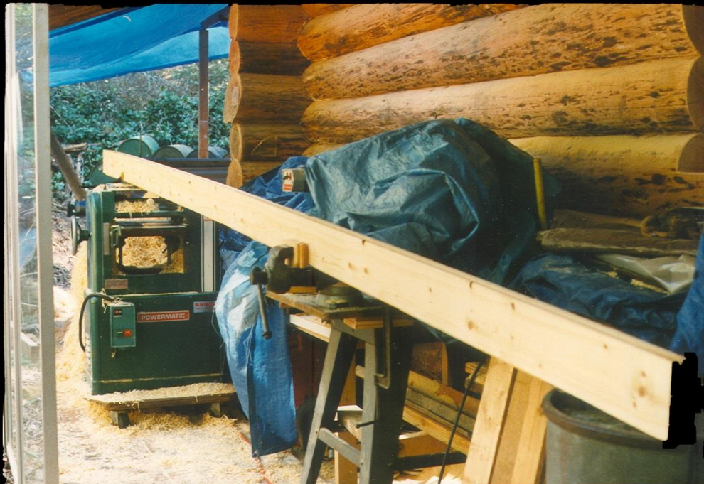
Setup For Planing Chamfers With Electric Hand Planer After Resurfacing And/Or Depending On Which Side Of Board Was Chosen, A Chamfer Would Most Likely Be Needed
