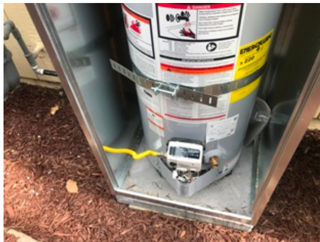
Unsafe Installation of Water Heater Gas Line
