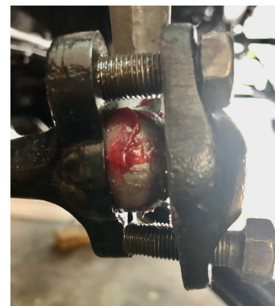
Drag link socket and ball arm cap filled with grease, and bolts fitted.
