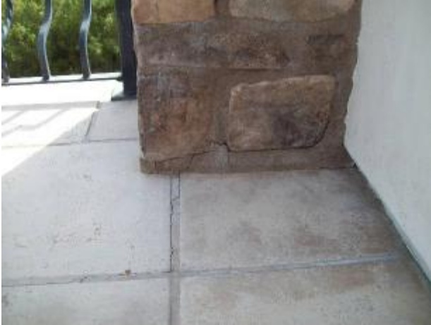
Cracks at the base of the NE handrail column at the balcony.
