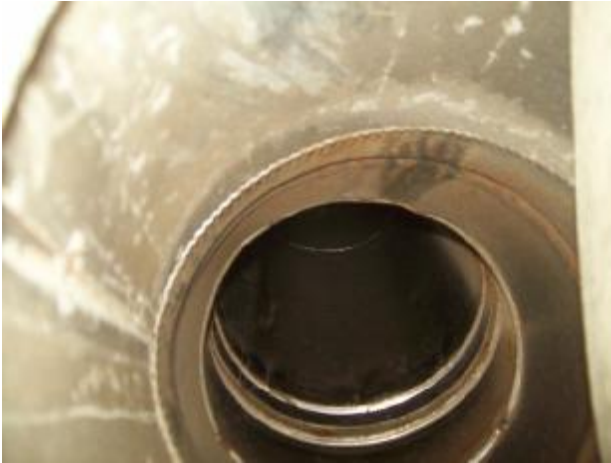
Gaps observed where the metal chimney attaches to the top of the firebox in the outdoor fire place.
