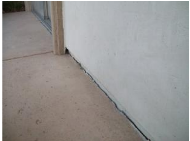
The concrete patio at the north side of the master suite has settled and pulled away from the home.
