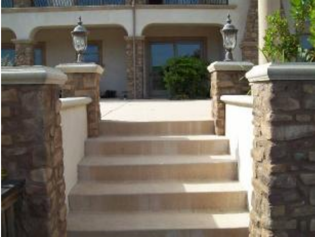
Hand railing is needed at the concrete stairs at the backyard patio area.
