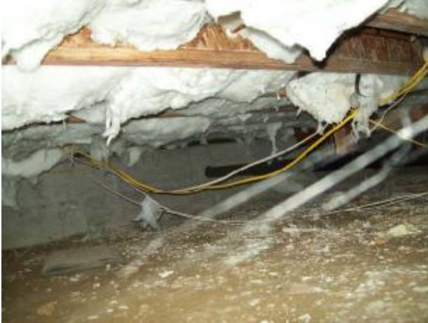
Unsecured wiring in the substructure area.
