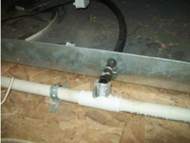
Substandard connection for the FAU condensate drain line to the A/C primary drain line.
