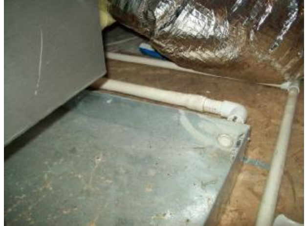
Improper installation of the propane pans below the furnaces in the attic.
