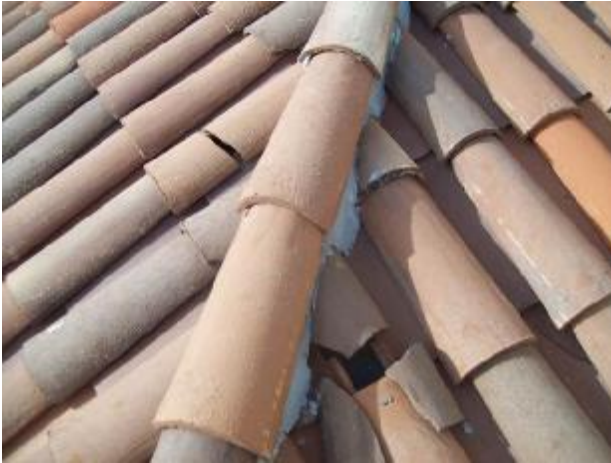
Cracked and displaced roof tiles at the hip above the garage.
