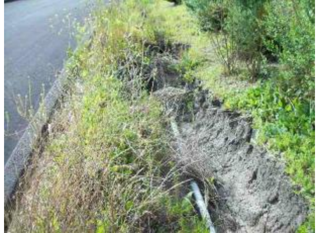
Erosion control is needed at the trench along the east property line.
