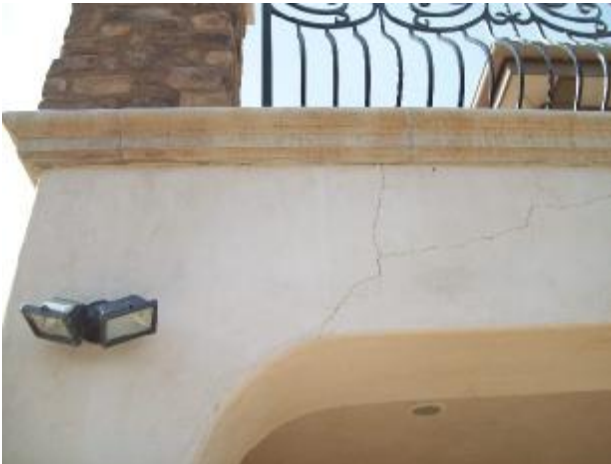
Differential crack in the stucco at the NE corner of the second story north side balcony.
