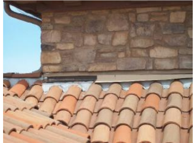
Partly damaged and partly missing roof-to-wall flashing above the garage.
