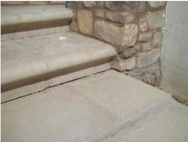
Settlement observed at the concrete patio at the east side of the front entry area.
