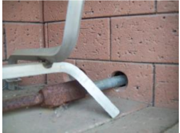
Noncombustible caulking is needed where the gas line penetrates the refractory plate in the outdoor F/Pl.
