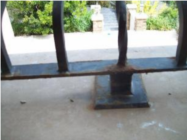
Example of some of the rusting at the wrought iron railings around the second story balconies.
