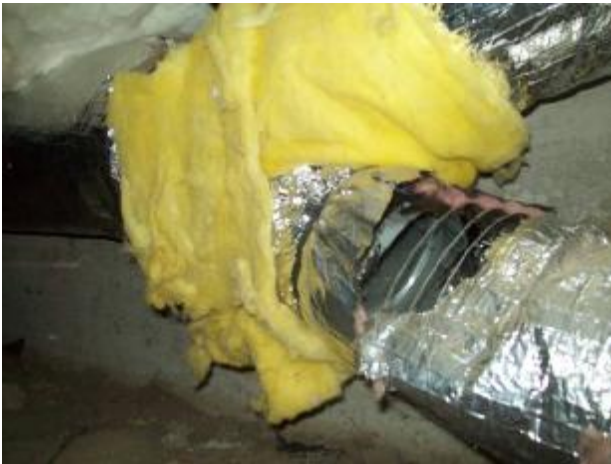
Damaged HVAC duct in the substructure area.
