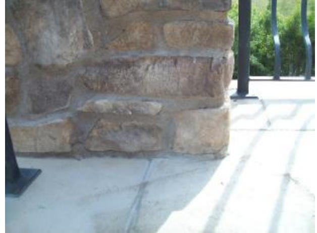
Cracks at the base of the SE handrail column at the balcony.
