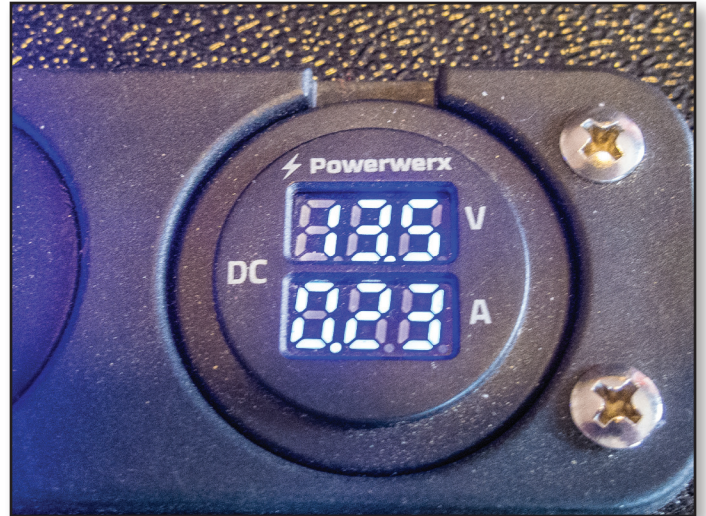
6. Volt/Amp meter on the battery box
