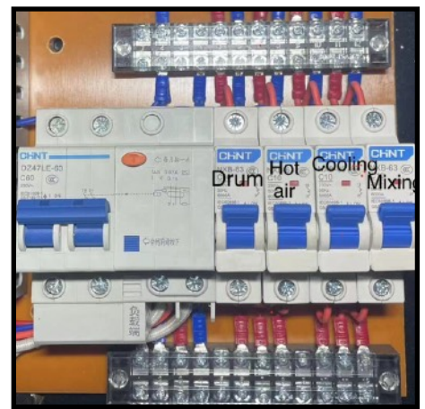
NEW CIRCUIT BREAKER SYSTEM
