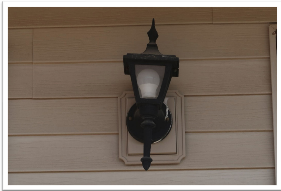
Photograph 27: Typical view of exterior light fixture
