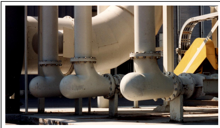
10" Smart Elbows™ in new high pressure system.
