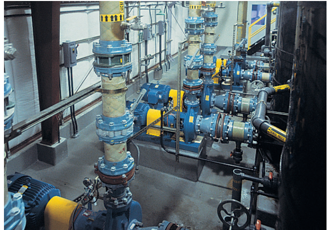
Multi-stage scrubber pump room.
