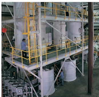
Multi-stage scrubber system (Tri-NOx) constructed of polypropylene and fiberglass, with catwalk access.
