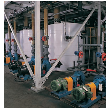
Multi-stage external recirculation system.
