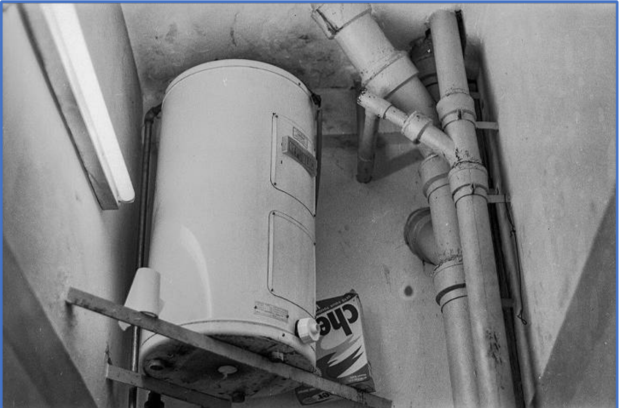
Bathroom Water Heater and Plumbing
