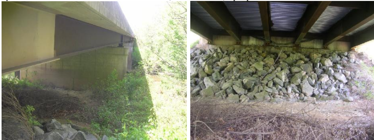
Figure IX.1 (left) Photo of the east pier on the upstream side of the Route 360 bridge over the Appomattox River. (right) Photo of the east abutment covered with 1' to 2' (0.31m to 0.61m) rip-rap. (AUR photos, April 24, 2013)
