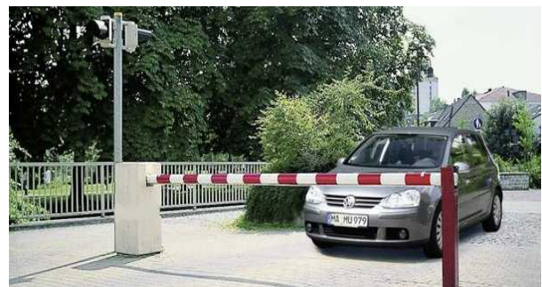
Parking Management: Comfortable access without waiting
