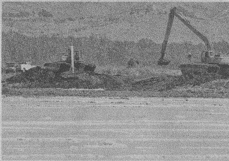
Amphibious excavators breach the levees to bring the Napa River flowing into the large salt pond near American Canyon.
