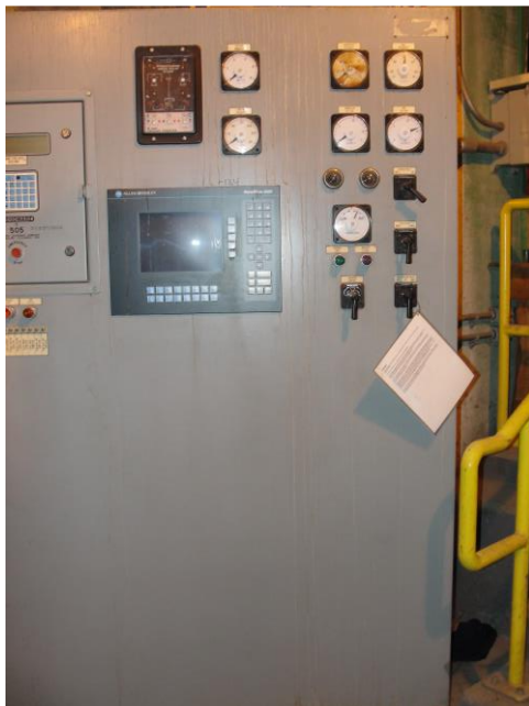
Turbine control panel
