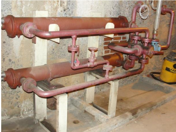
Lube oil Coolers
