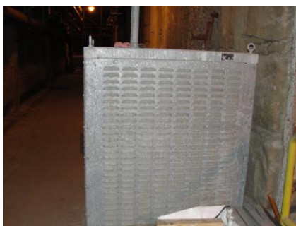
Neutral Ground Resister
