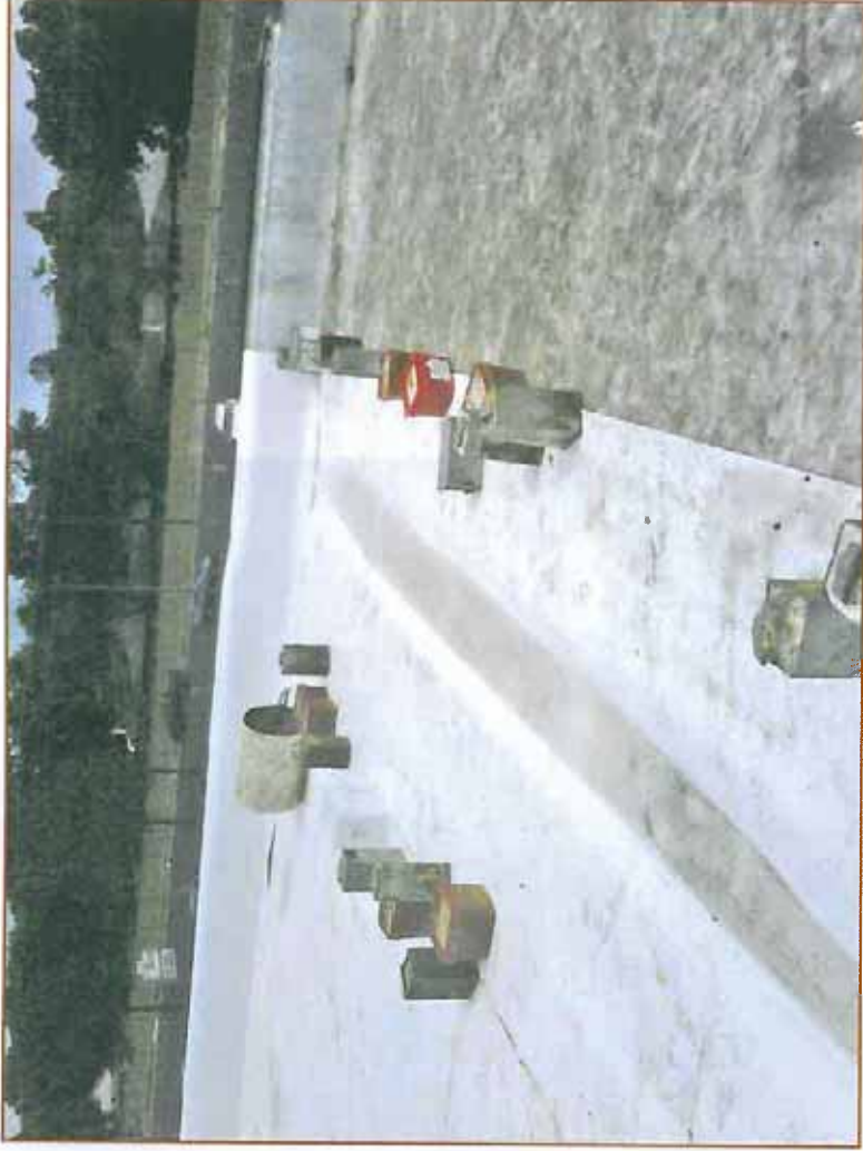
Photo 4 – Water accumulation on depression at tie-in.
