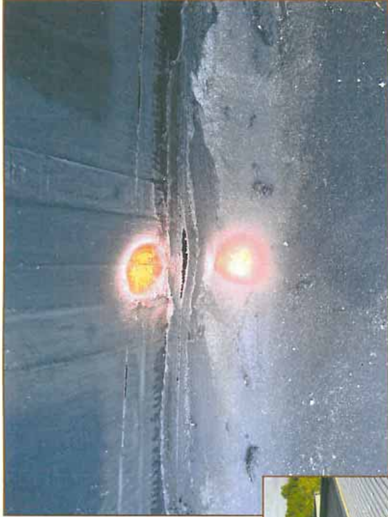
Photo 6 – Disbonded felts along parapet wall.
