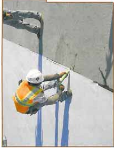
Photo 13 – Sealant applied along edge of fleece-backing single ply over lightweight insulating concrete.
