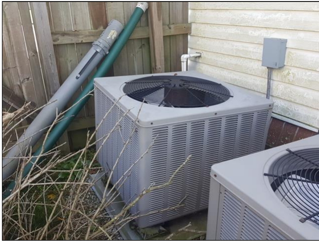
heat pump/right side of home
