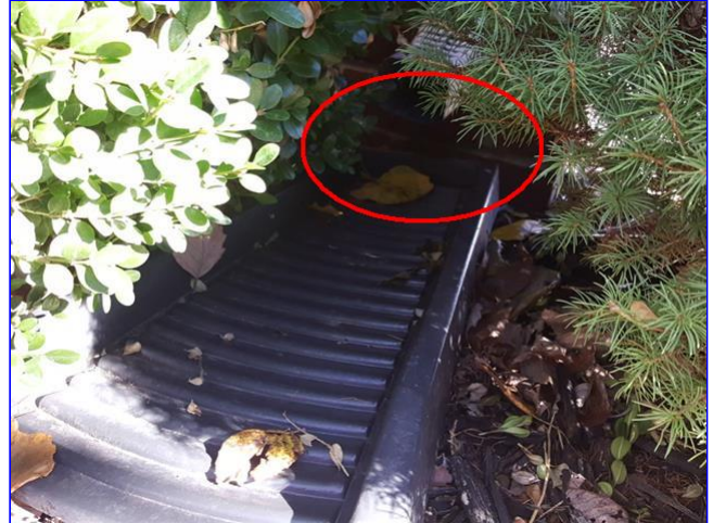
2.3 Item 9(Picture) front left corner of garage
