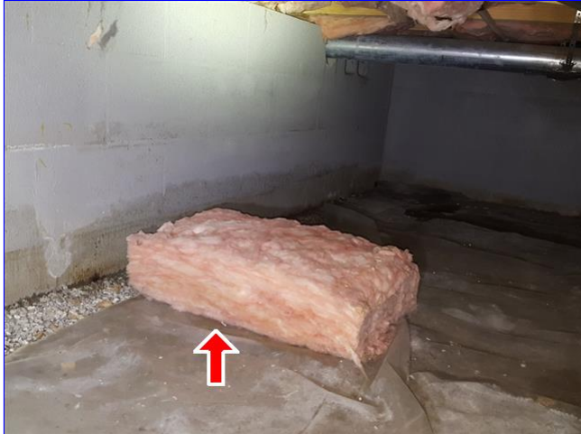
1.3 Item 1(Picture) under master bathroom area
