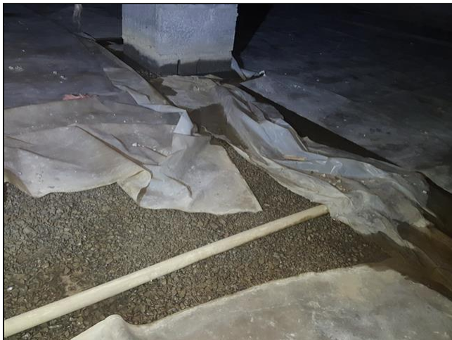
1.3 Item 6(Picture) under dining room area
