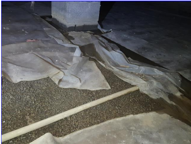
1.3 Item 6(Picture) under dining room area
