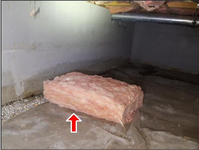
1.3 Item 1(Picture) under master bathroom area
