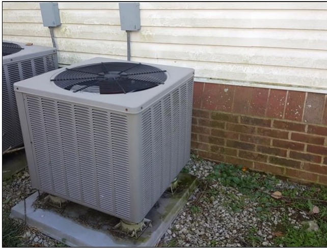
heat pump/right side of home
