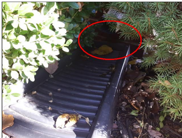
2.3 Item 9(Picture) front left corner of garage
