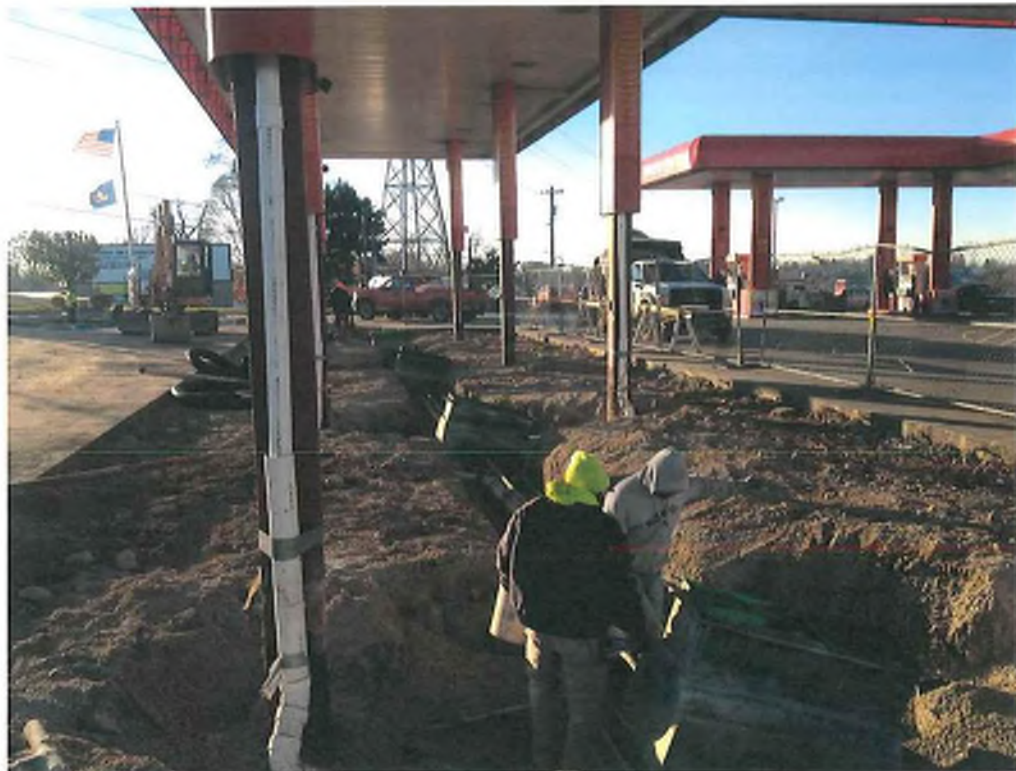
View of pumps 1 through 10 facing south/southeast
