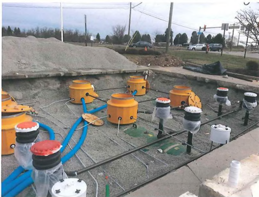
New tank top equipment
