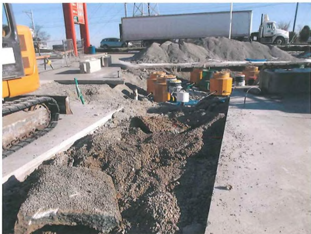
Product line trench and tank top equipment
