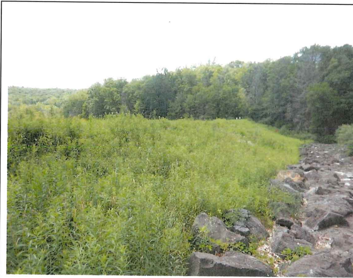
7. View of the downstream slope from the right abutment. Note the tall grass.
