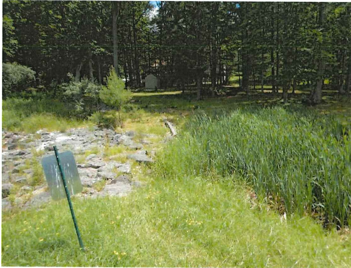
11. View of the inlet of the auxiliary spillway channel. Note the cattails at the inlet.
