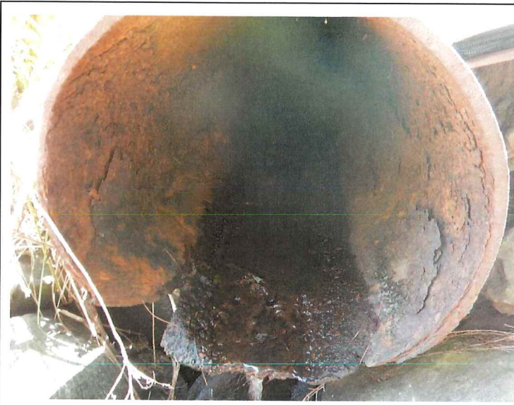
10. View inside the principal spillway discharge pipe. Note the scaling of the metal.
