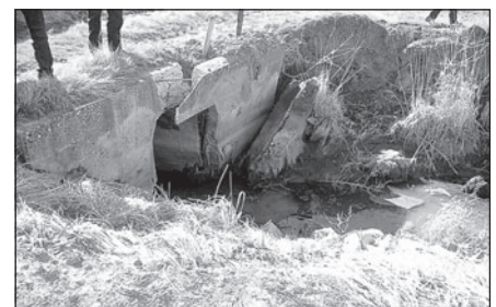
Crumbling Concrete Structure
