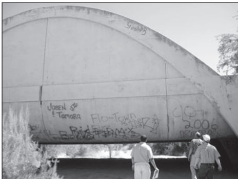
Deteriorating China Wash Flume
