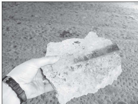
Source: GAO. Concrete that Fell from Flume
