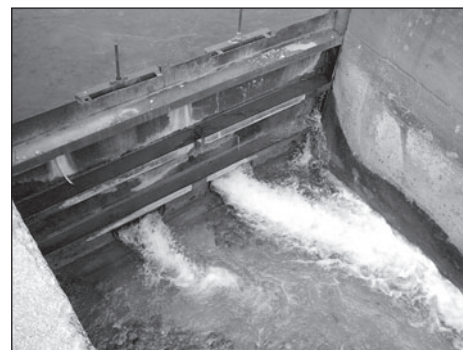
Leaking Check Gate
