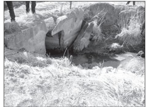
Crumbling Irrigation Structure
