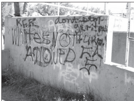
Source: GAO. Graffiti on Irrigation Structure
