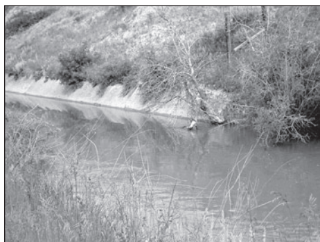
Source: GAO. Deteriorating Canal Lining
