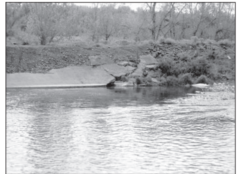
Irrigation Canal with Crumbling Concrete Lining
