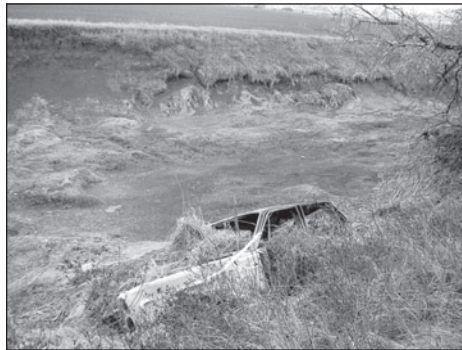
Source: GAO. Abandoned Car in Deteriorated Canal
